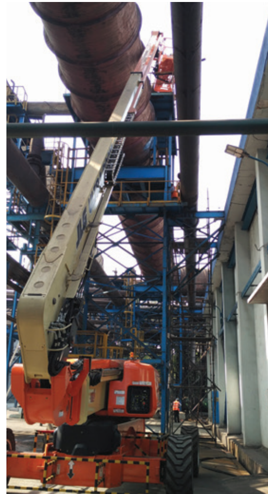
Major pipeline maintenance carried out by United Express at the Jamshedpur plant.
